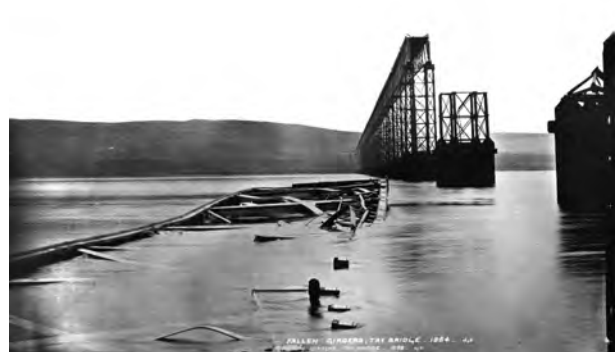
5 Side of the high girders seen at low tide. The girders were found almost intact close to the pier bases, and laid out in a wave form alongside the high section of the bridge
