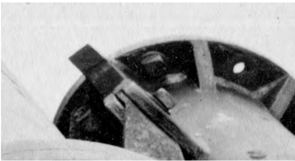
12 Conical taper on broken strut lug with intact upper lug joint in foreground
