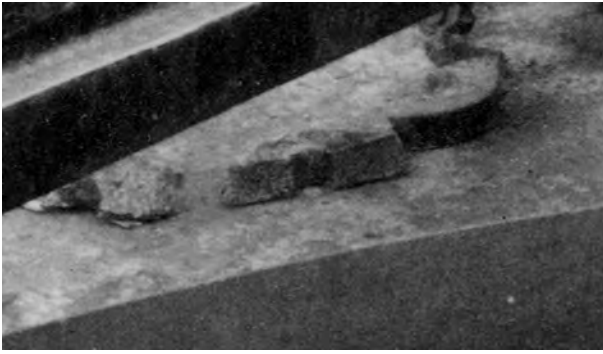
13 Closeup of three broken lugs from twelfth pier. The centre sample shows numerous crack arrest lines with a small blowhole on the lefthand wing of the lug, probably indicating intermittent crack growth (fatigue)
