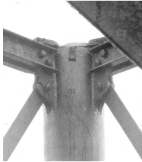
14 Closeup of fractured lug on third pier (looking west). Only one wing of the lefthand lug has broken, suggesting cyclic loading during or before the accident and collapse of the tower. There are no washers on the strut bolts, and these appear to be tightened by different amounts (judging by differing thread heights above the nuts)
